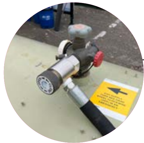
Shut off valve – for operational and emergency use
