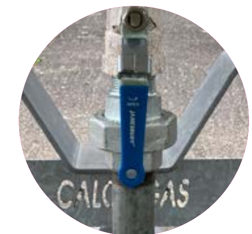
Shut off valve for operational and emergency use
