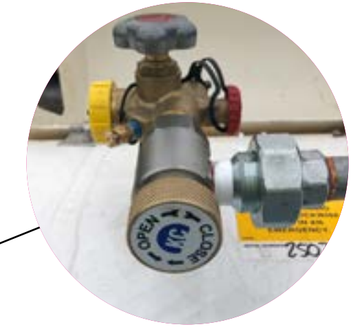
Bypass return and emergency isolating valve
