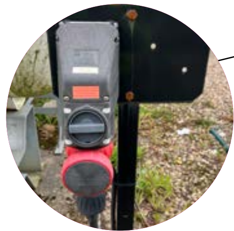
Electric pump control switch
